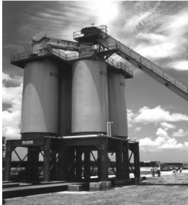
Figure 11.4 Stationary five bin silo system.
