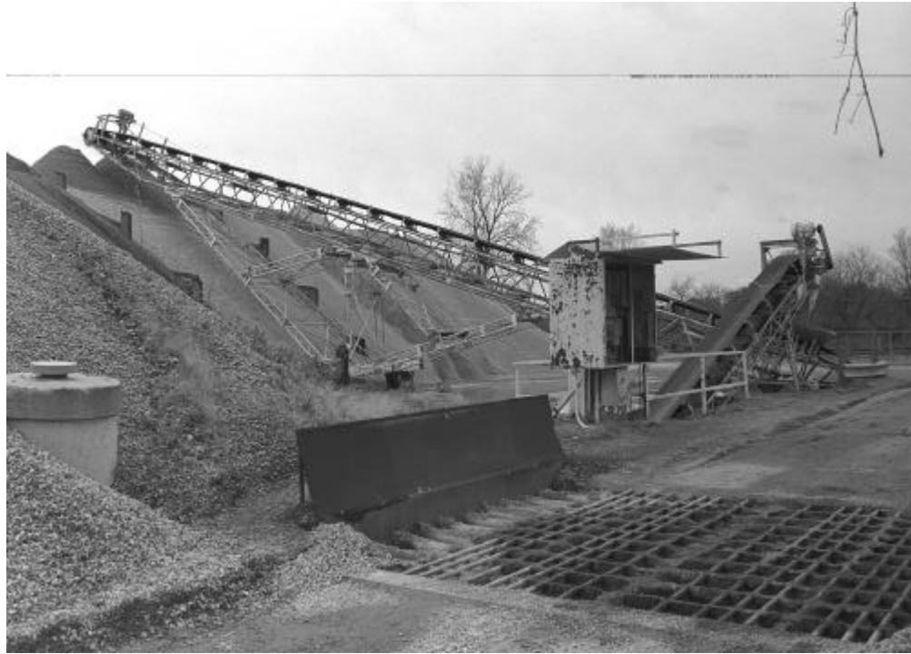
Figure 3.5 Radial stackers at quarry facility.
