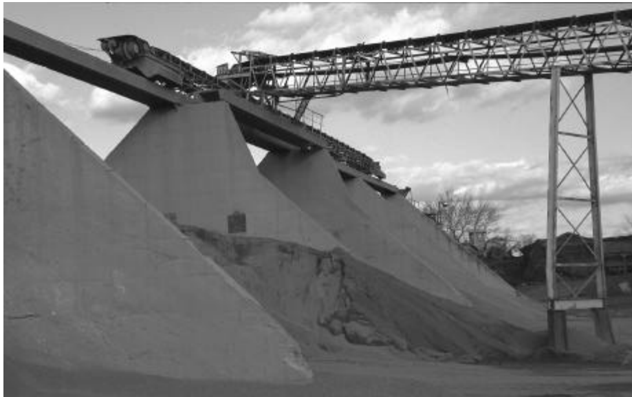
Figure 3.7 Bunker storage with rail off-leading system.
