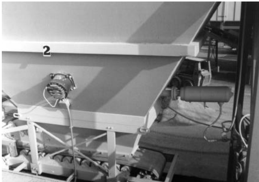
Figure 3.35 Bin wall vibrators and air cannon on cold feed bin.
