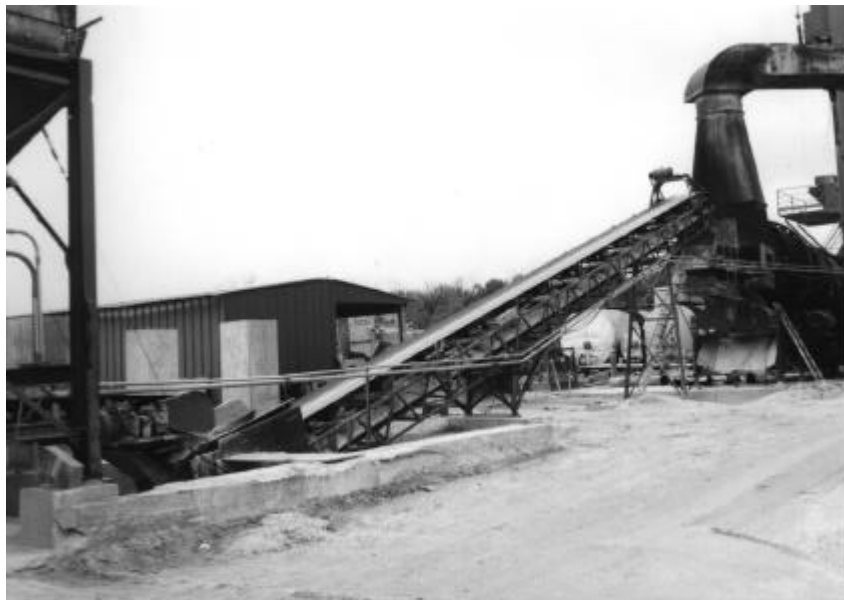
Figure 3.41 Dryer feed conveyor on batch plant.
