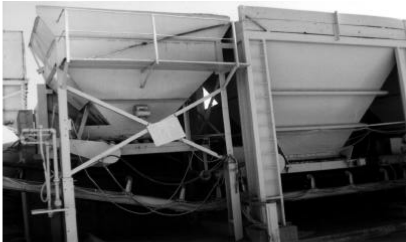
Figure 3.45 Dust bin at the end of a cold feed system.
