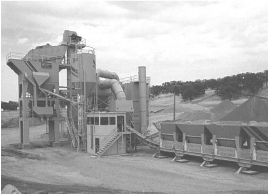
Figure 3.25 Batch plant with feeder belts on cold feed bins.
