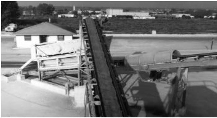
Figure 3.43 Double deck scalping screen on drum-mixer with air operated deck selector.
