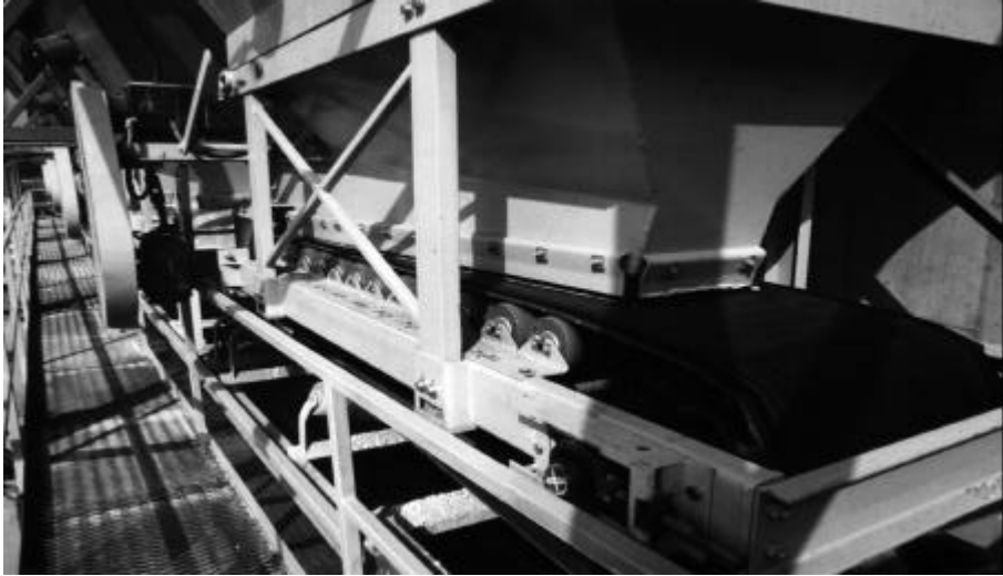
Figure 3.31 Feeder belt and hopper showing trapezoidal shape to opening.
