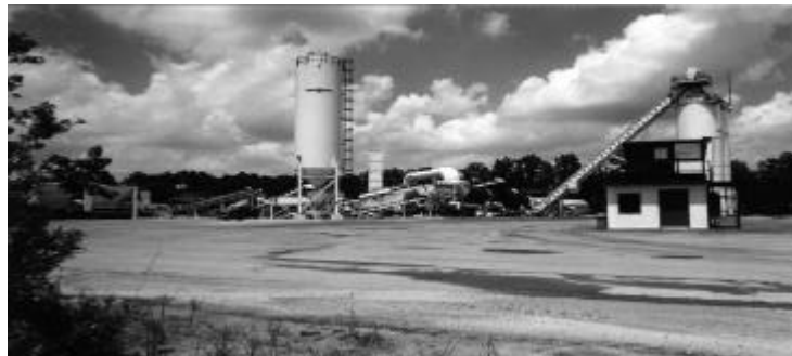
Figure 3.46 Lime silo sitting over a belt conveyor.
