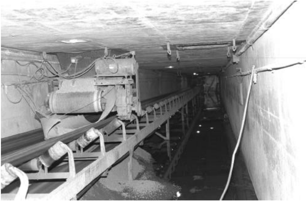
Figure 3.8 Belt feeder below bunker storage.
