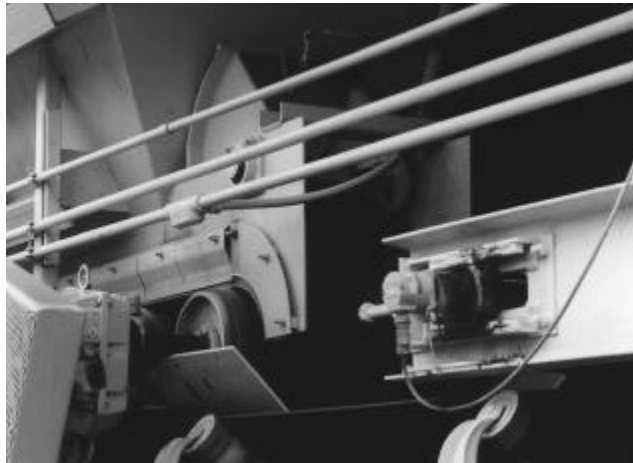
Figure 3.36 Tachometer on tail shaft of feeder to detect belt slippage or breakage.
