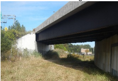
Re-Use Existing OLRFM over WSSC waterline to maximize project scope. The existing bridge is excellent condition.
