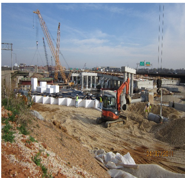
EPS Geofoam used on Facchina's 11th Street Bridge Project in Washington, DC to achieve zero-net loading on critical utilities.
