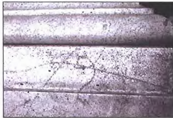
Very high-pressure water has scarred this granite. Photo: NPS files.
