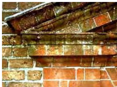
This 18th century pediment and surrounding wall exhibit distinctively different mortar joints. Photo: NPS files.
