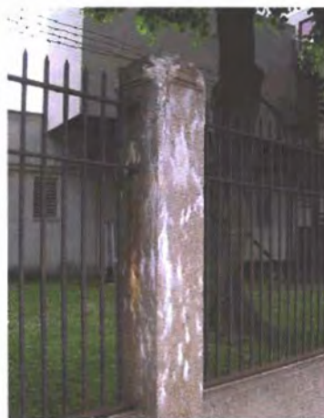
Figure 15. Evidence of moisture movement through concrete is apparent in the form of mineral deposits on the concrete surface. Cyclic freezing and thawing of entrapped moisture, and corrosion of embedded reinforcement, have also contributed to deterioration of the concrete column on this fence at Crocker Field in Fitchburg, Massachusetts, designed by the Olmsted Brothers.
