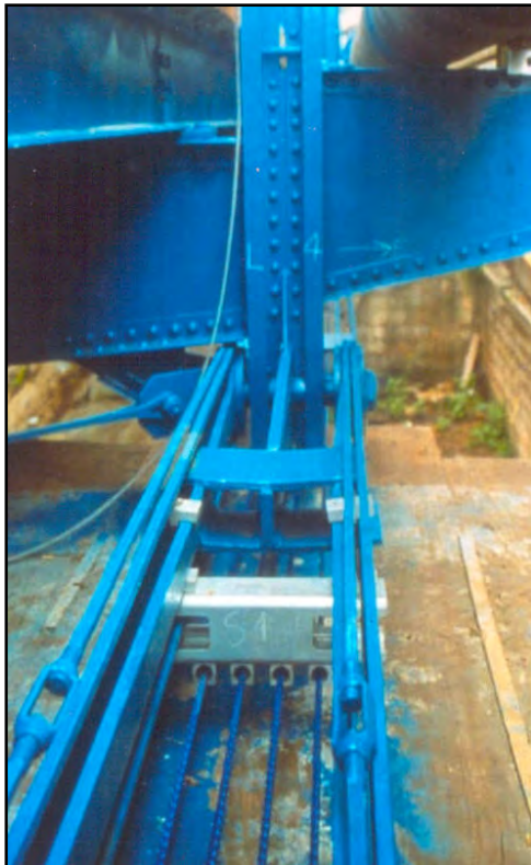
Figure 4 (left). Post-tensioned lower chord of pin-connected thru truss bridge. Note new members and guide placed between the eyebar packs.
