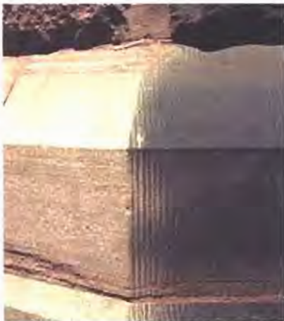
On the left, grit blasting has obliterated the vertical tooling marks from granite, a very dense stone. Photo: NPS files.
