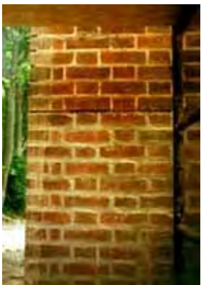
A mechanical grinder improperly used to cut out the horizontal joint and incompatible repointing have seriously damaged the 19th century brick. Photo: NPS files.
