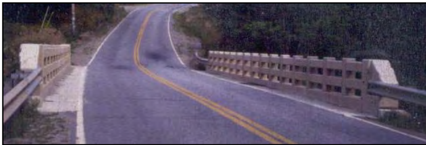
Figure 8. Partridge Bridge, Maine, an example of new railings, inspired by, but not exact replicas of, the original. Note the detail for the acceptable attachment for the approach guide rails.
