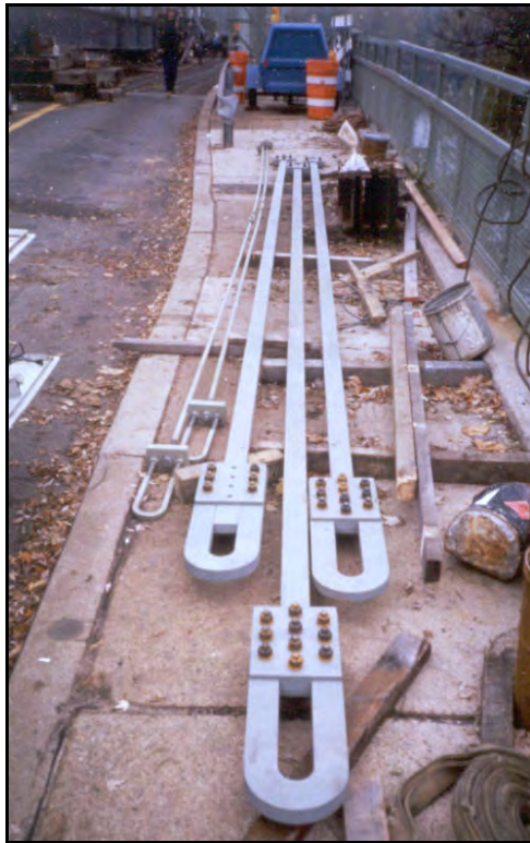
Figure 2 (below). Use of high-strength bolts to replace rivets. It is best to specify to which side to place the heads and the shanks to ensure a consistent appearance. In this example, some shanks are on the wrong side.
