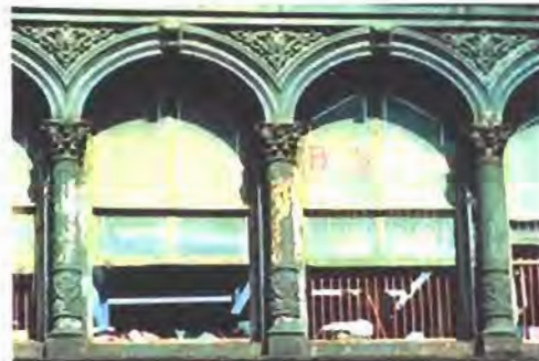
Cast iron may be abrasively cleaned, but must be painted immediately to prevent rust. Photo: NPS files.
