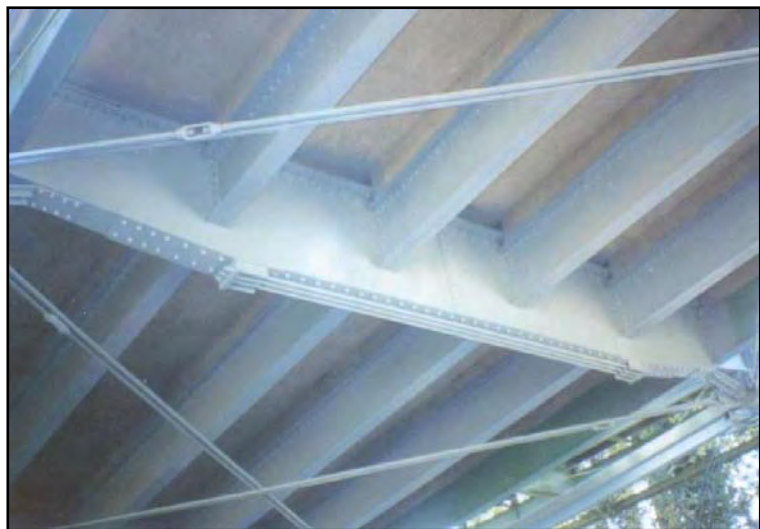
Figure 5 (below). Post-tensioned floorbeam using standard high-strength rods. This increases the capacity of the floorbeam.
