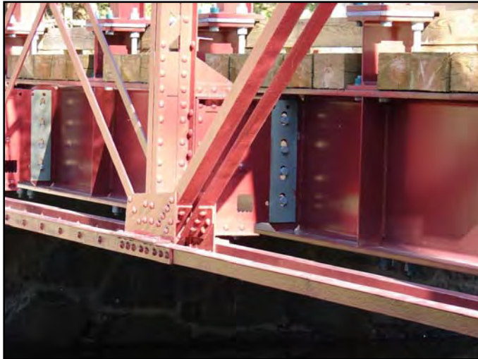
Figure 6. When attaching historic truss lines to a new superstructure make sure to retain a sufficient length of the floorbeams to facilitate attachment to the beams. The truss lines support themselves.
