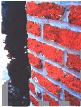
Abrasive cleaning can cause permanent damage to historic fabric, such as this brick wall. Photo: NPS files.
