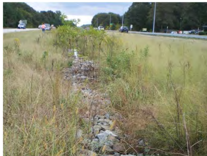
Excessive Vegetation in Infiltration Trench
