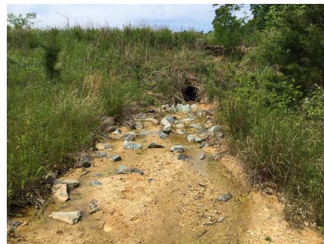
Major Sediment Accumulation at Outfall
