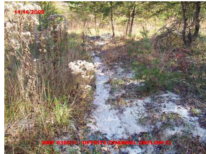
Minor Sediment Accumulation in Inflow Ditch
