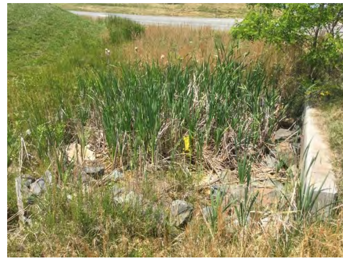
Vegetation Growing in Riprap
