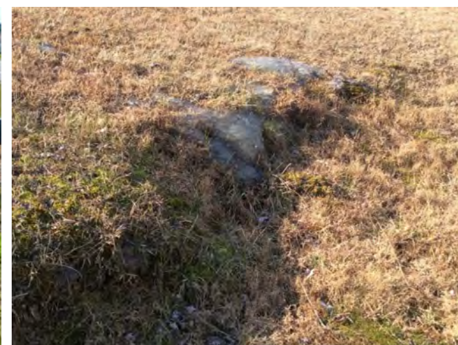
Frozen Seepage Through Embankment
