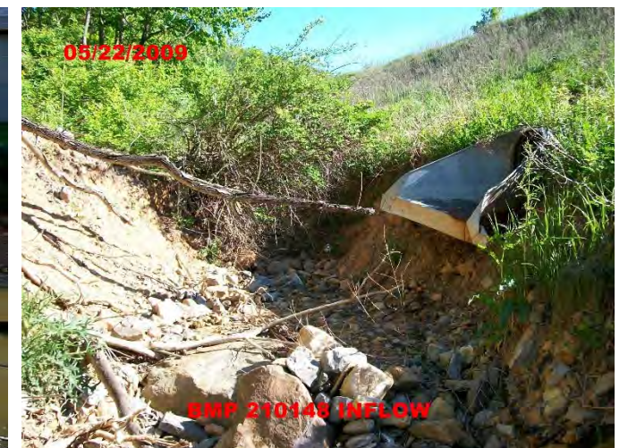
Major Erosion at Inflow Point
