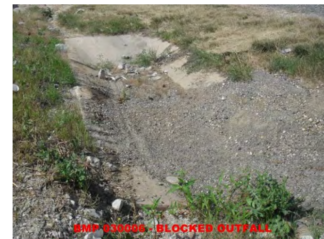
Accumulated Sediment Blocking Outfall Point
