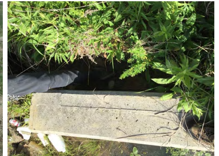
Minor Erosion Behind End Structure
