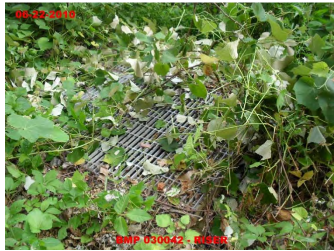
Vegetation Obstructing Outflow Point
