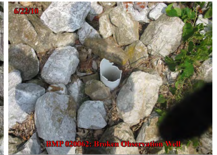
Broken Observation Well
