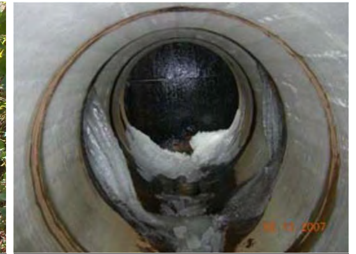
Water Leaking into Pipe
