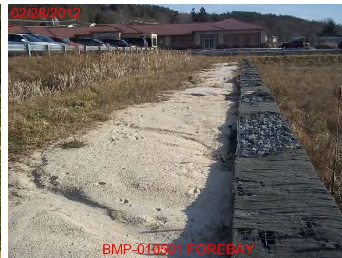
Major Sediment Accumulation in Forebay
