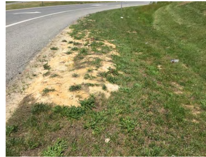
Small Area of Bare Soil in Grass Swale
