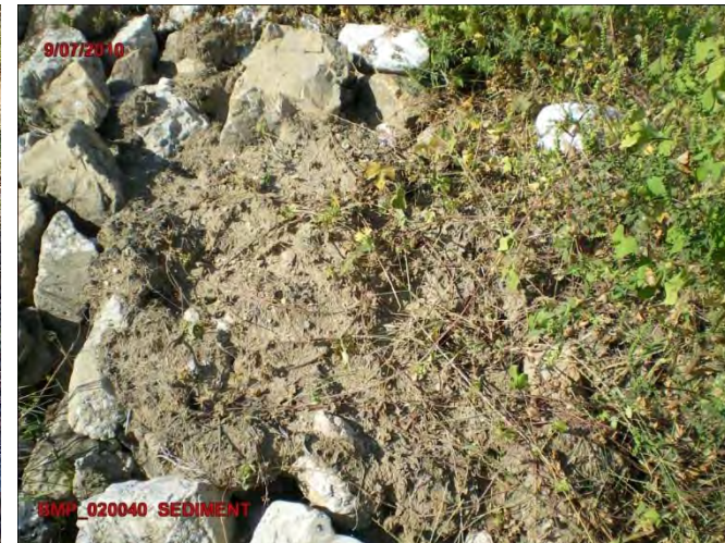
Minor Sediment Accumulation
