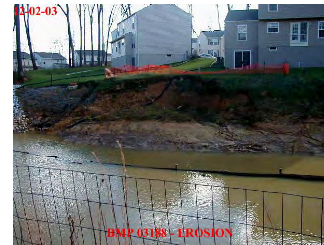
Major Erosion Along Pond Bank
