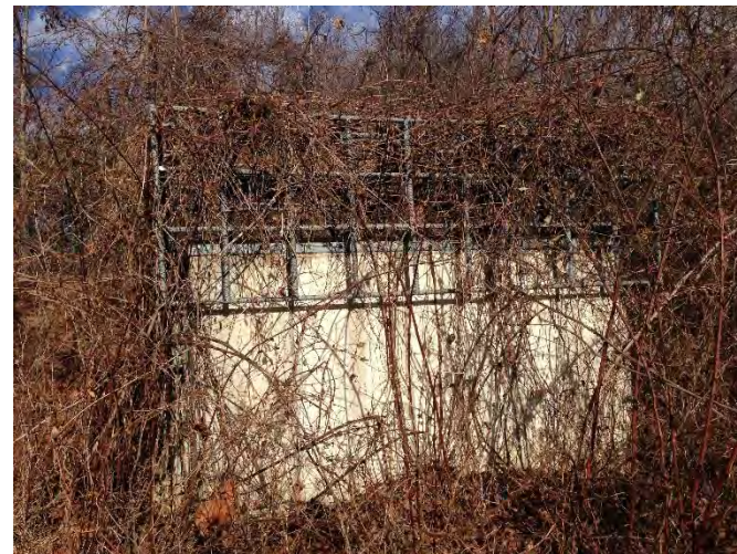
Vegetation Obstructing Riser Structure
