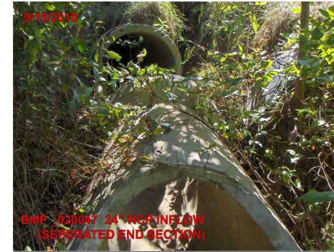
End Structure Separated From Pipe
