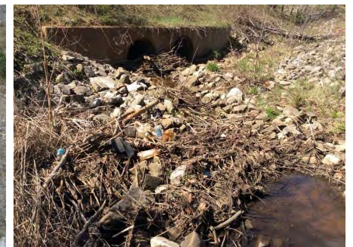
Accumulated Debris Blocking Outfall Point
