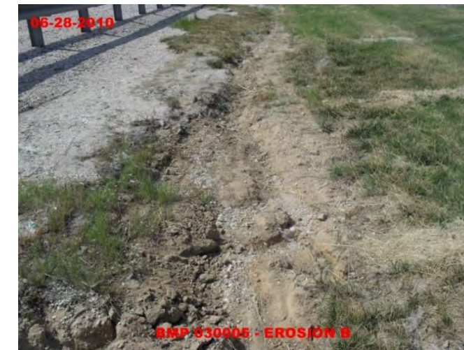
Minor Erosion in Grass Swale
