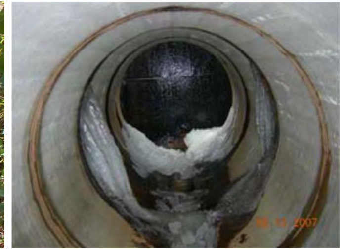
Water Leaking into Pipe
