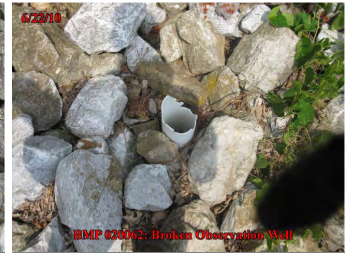
Broken Observation Well
