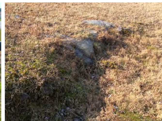
Frozen Seepage Through Embankment
