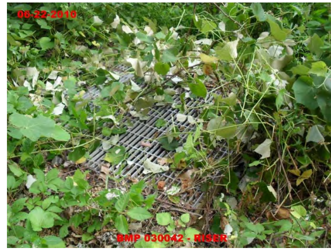
Vegetation Obstructing Outflow Point
