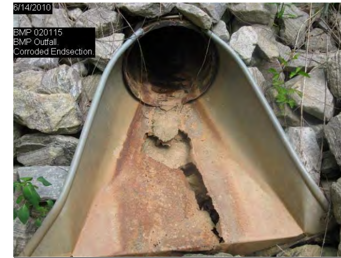
Deteriorated CMP End Structure
