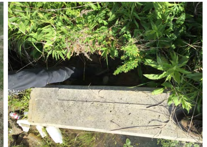
Minor Erosion Behind End Structure
