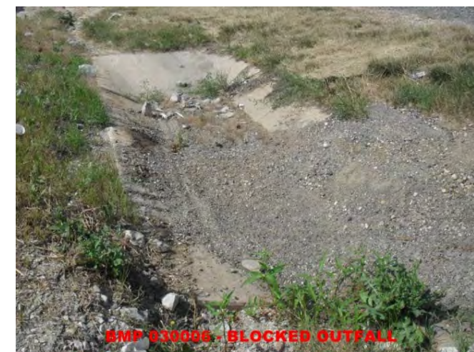
Accumulated Sediment Blocking Outfall Point
