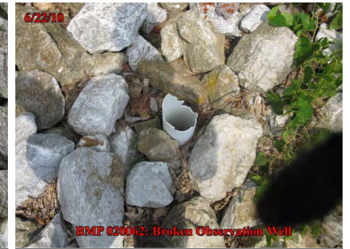
Broken Observation Well
