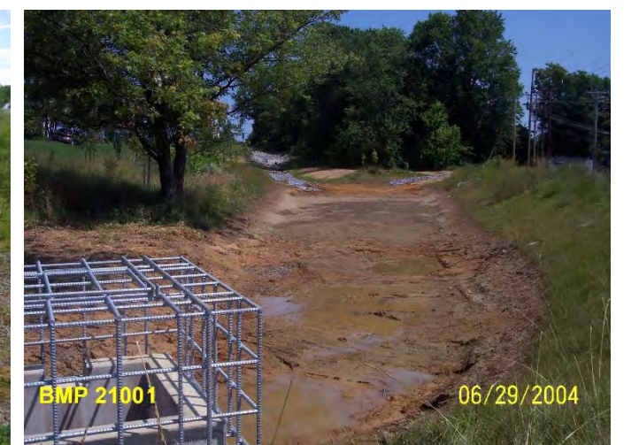
Large Area of Bare Soil on Pond Bottom
