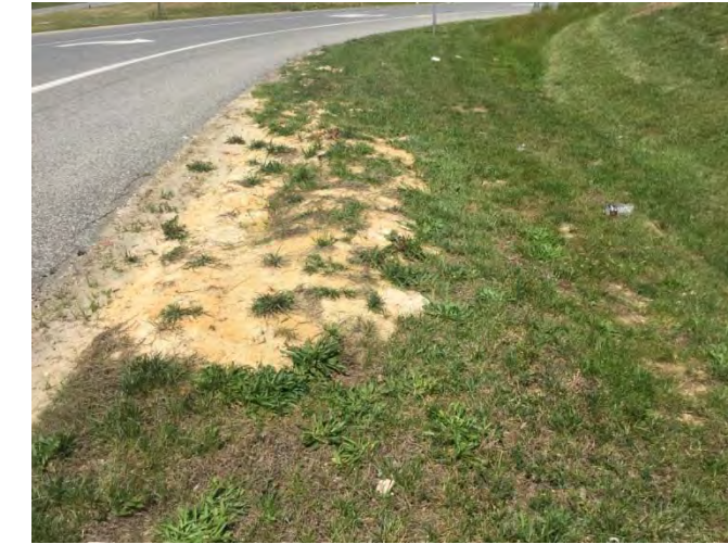
Small Area of Bare Soil in Grass Swale
