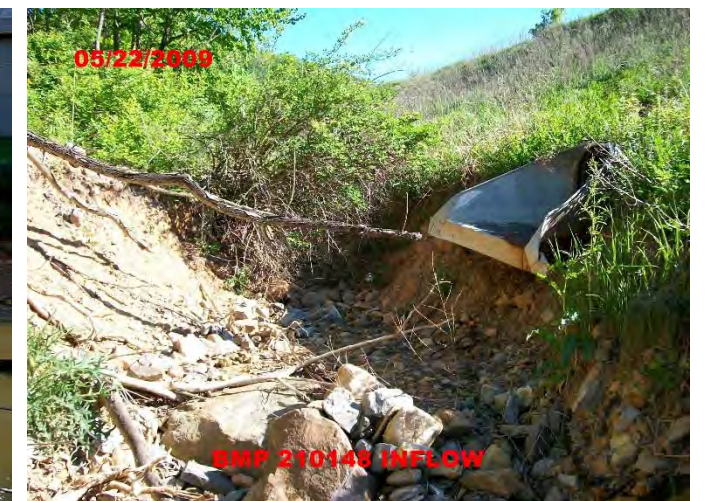
Major Erosion at Inflow Point
