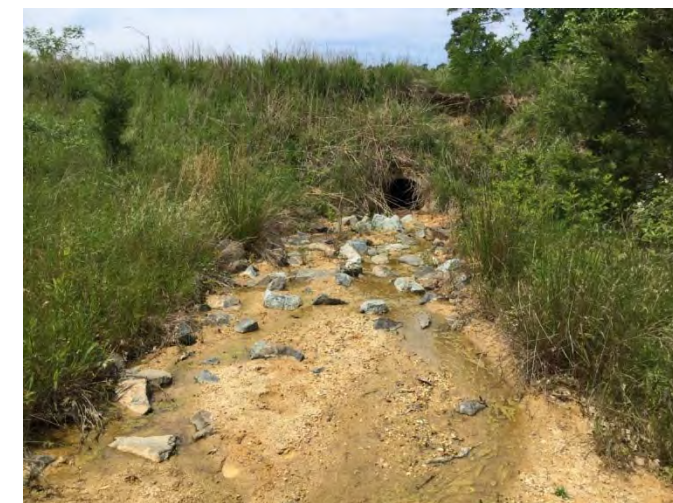
Major Sediment Accumulation at Outfall
