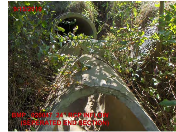
End Structure Separated From Pipe
