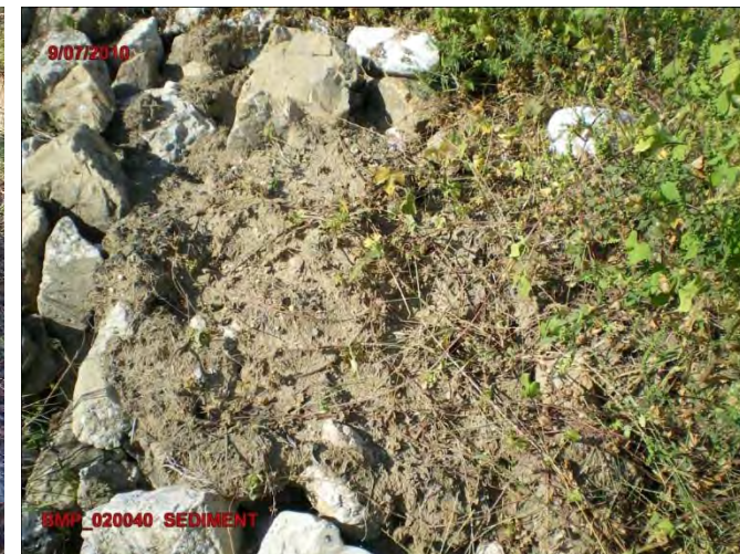
Minor Sediment Accumulation
