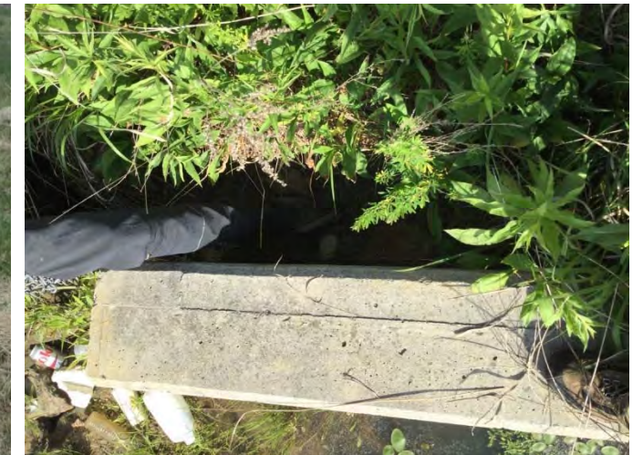
Minor Erosion Behind End Structure
