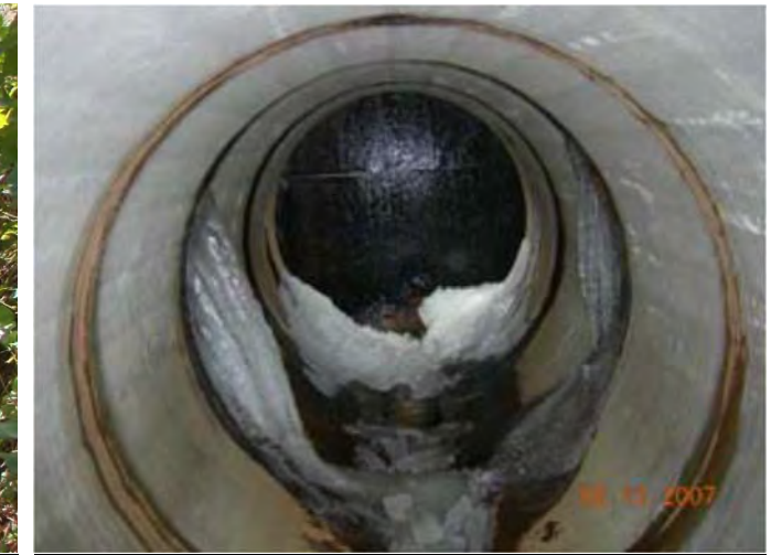
Water Leaking into Pipe
