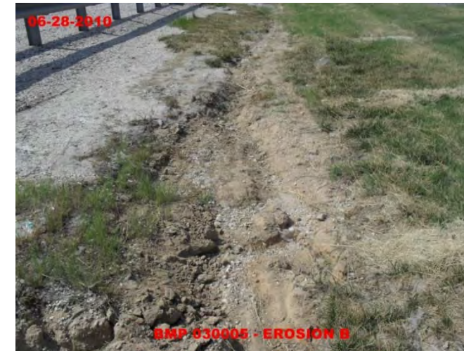
Minor Erosion in Grass Swale
