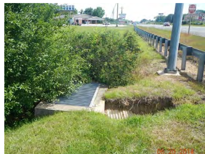
Eroded Embankment Exposing Pipe
