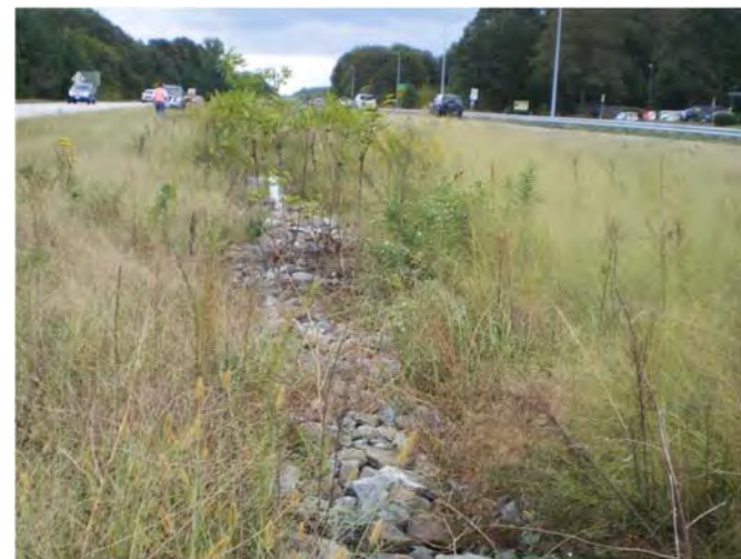
Excessive Vegetation in Infiltration Trench
