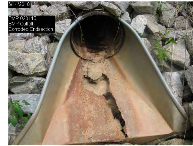
Deteriorated CMP End Structure
