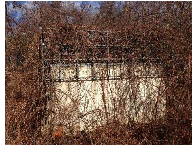
Vegetation Obstructing Riser Structure
