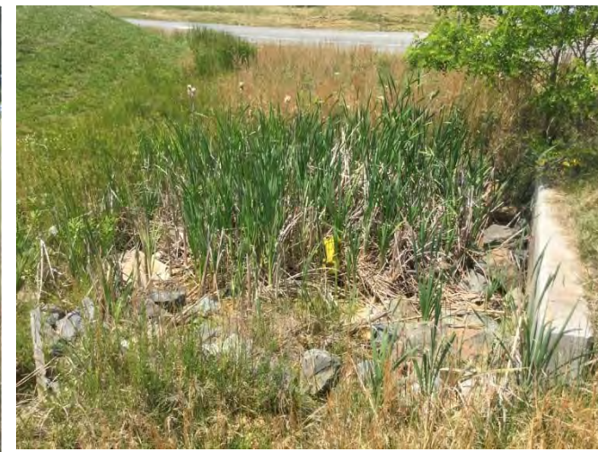
Vegetation Growing in Riprap
