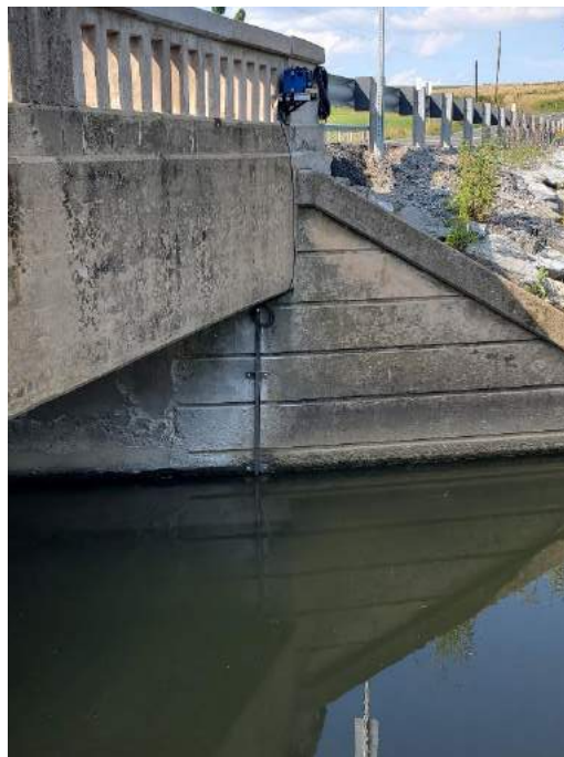
Figure 5. FY23 upstream station (Site ID 01636845) on Little Catoclin Creek near Rosemont, MD. The photo shows the ISCO velocity and area flow module.
