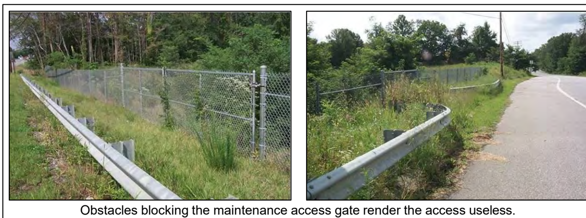
Figure 6-1. Obstructed Maintenance Access
