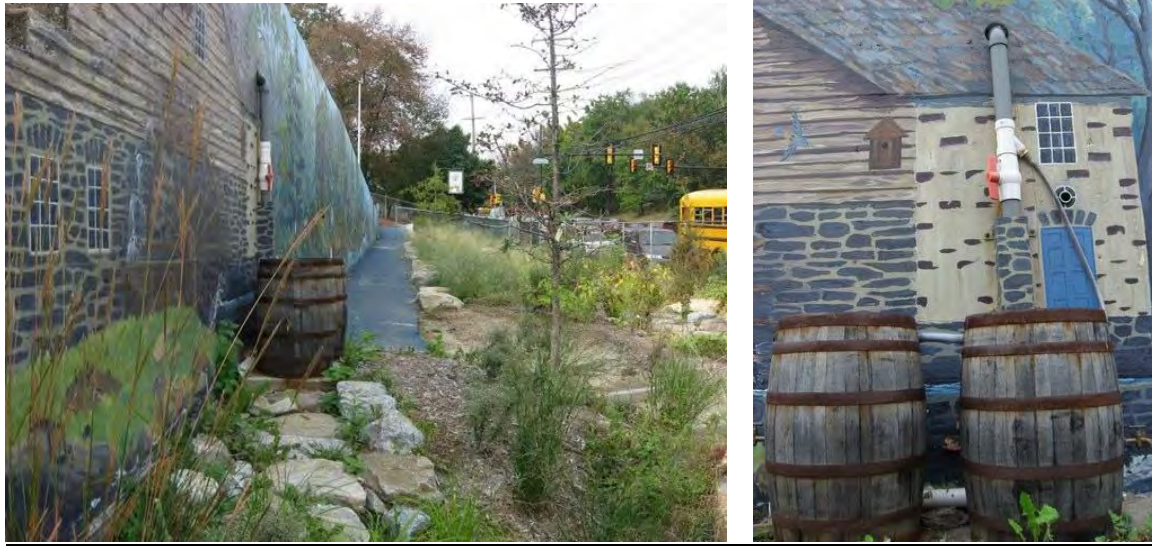
Rain Barrels collecting rooftop drainage
