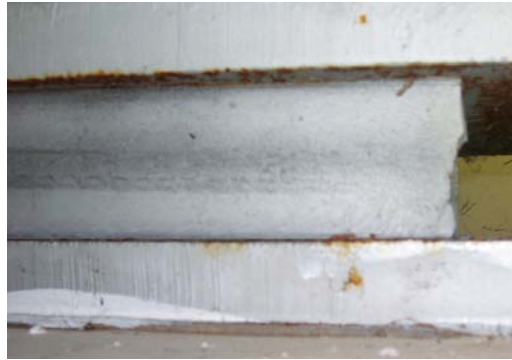
Figure 3.1 - Pad Deterioration in Bridge #1169
