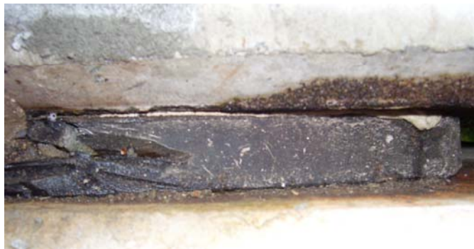
Figure 3.9 - Deterioration Due to Poor Quality
