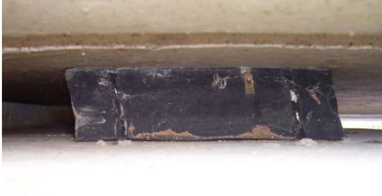
Figure 3.7 - Bulging in a Laminated Bearing
