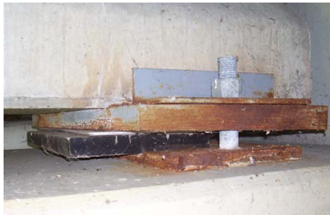
Figure 3.2 - Bearing Slip in Bridge #9015
