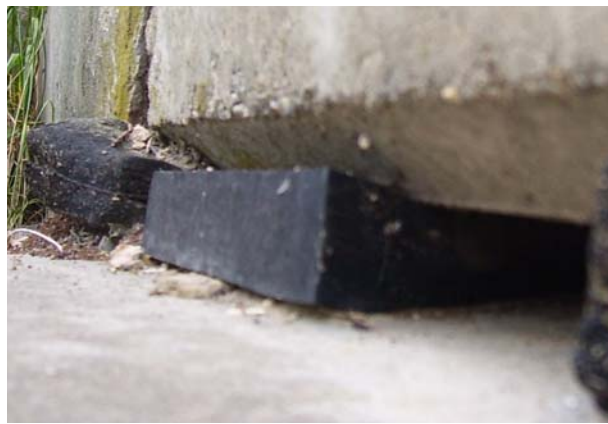
Figure 3.10 - Crushing in a Slab Bridge
