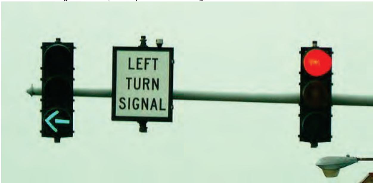
Protected left turn signal enforces protected left turns (Photo from Flickr - Benny Mazur)
