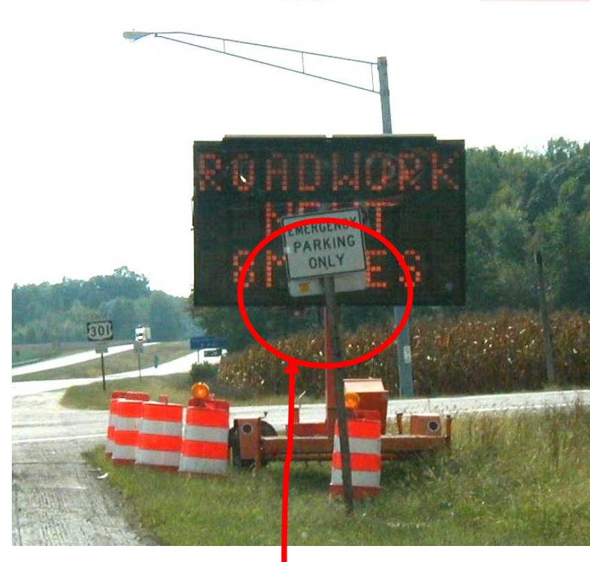
Unacceptable PCMS Placement
