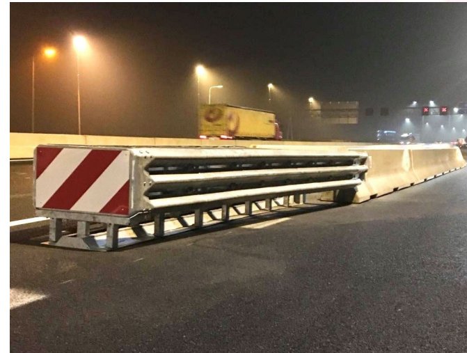
Re-directive W-beam crash barriers
