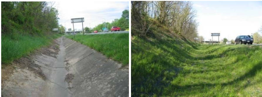
Figure 1-13: Before and After image of a Concrete Ditch Removal along I-70 in Washington County
