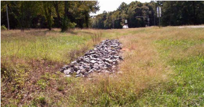
Figure 1-11: Infiltration Trench along US 113 in Worcester County
